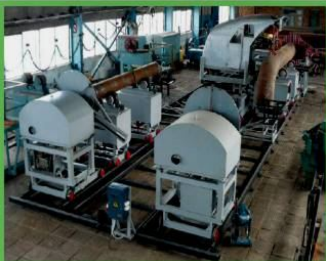
The general appearance of the installation
